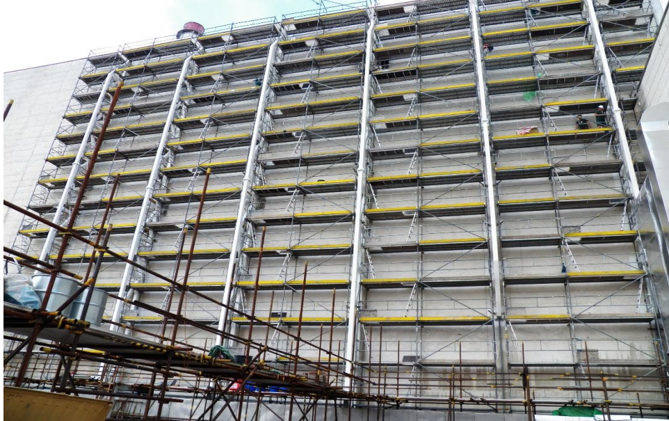
Figure 7. Reinforcement of the columns from the external part of the reactor building
