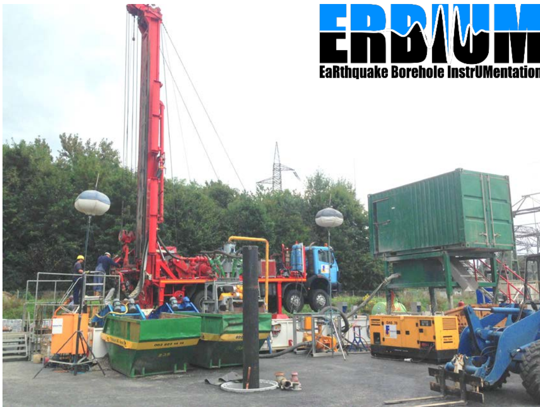
Figure 1. Construction work for drilling the boreholes and visible casing for one borehole in the front before shortening to ground level.
