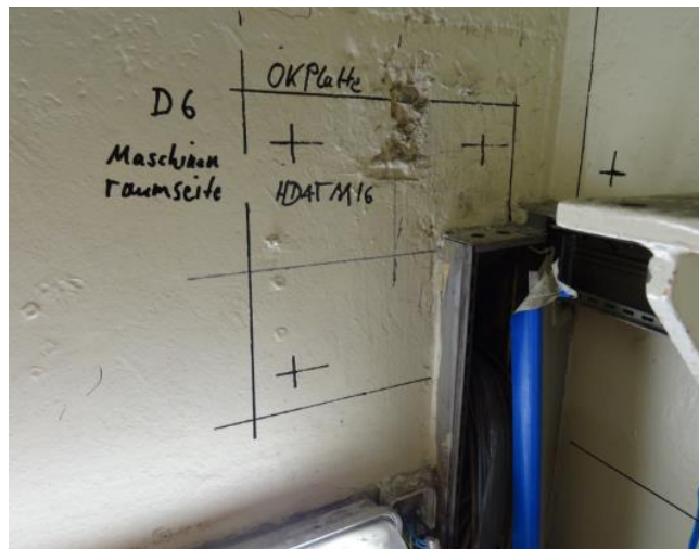
Figure 7. Cable duct as an interfering edge
