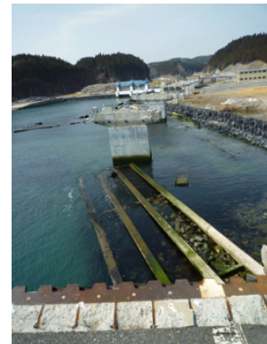
Photo 3 All bridge girders carried away by Tsunami
