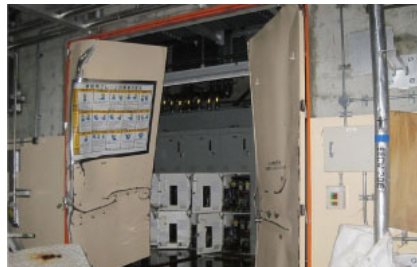
Photo 2 The electric apparatus which was destroyed by the water Pressure
