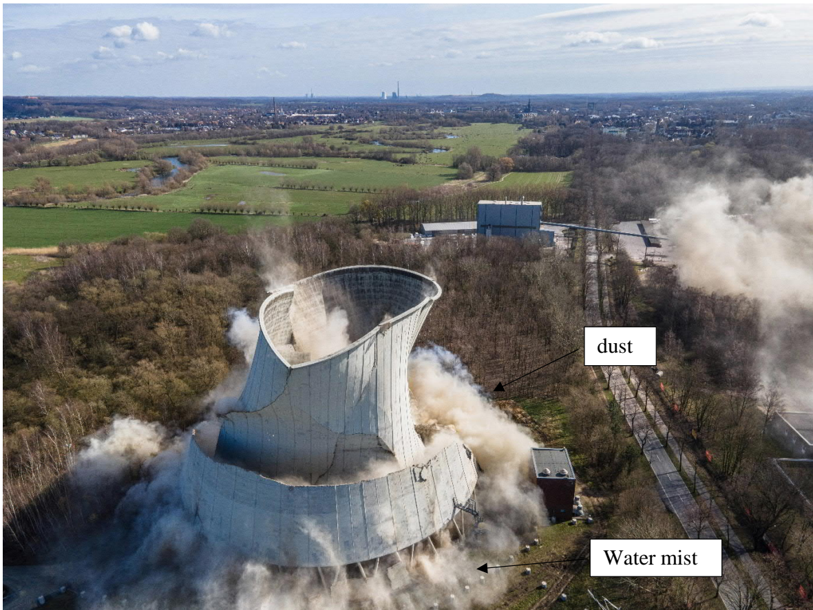
Figure 5: Collapse of the cooling tower at the power plant Luenen (Germany) (source: Fa. Hagedorn)
