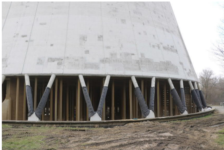
Figure 4: Covering the blasting zones of the columns of the cooling tower at the power plant Luenen (Germany)
