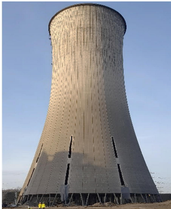
Figure 6: Pre-weakened cooling tower with three vertical slits at Knepper power station (Germany)
